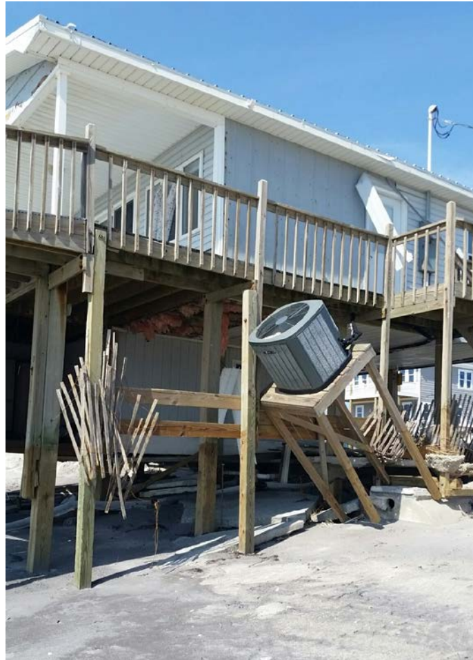
Figure 10: Property in North Topsail Beach with erosion and surge-induced property damage, note loss of vinyl siding though soffits and metal roof performed well.
