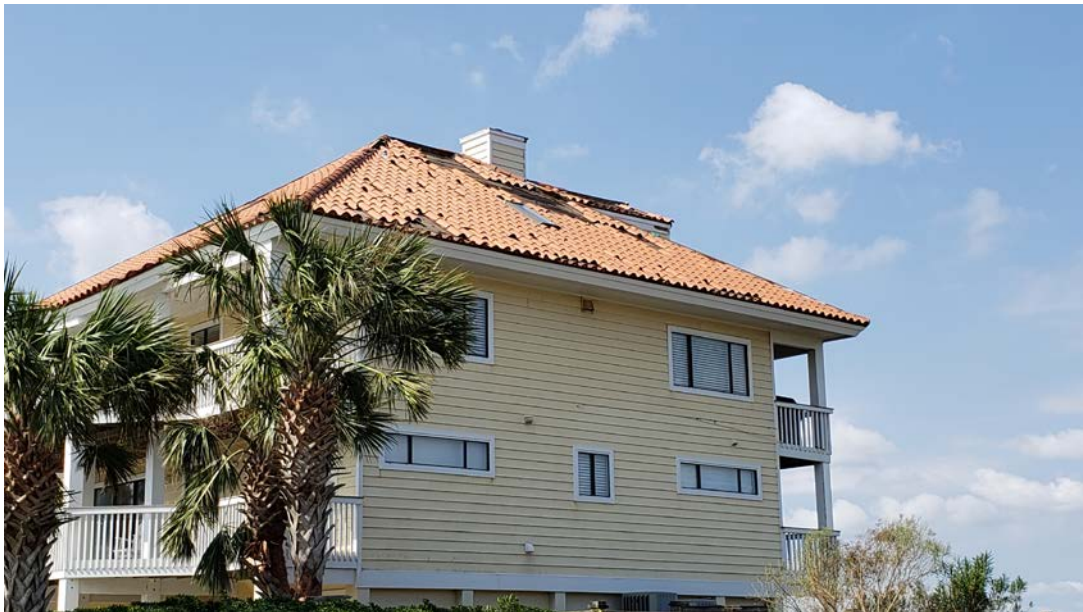
Figure 13: Damage to tile roof in Wrightsville Beach
