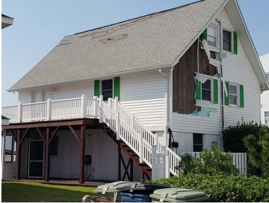
Figure 9: Loss vinyl siding installed over wood panel siding and shingle loss near roof ridge in Emerald Isle
