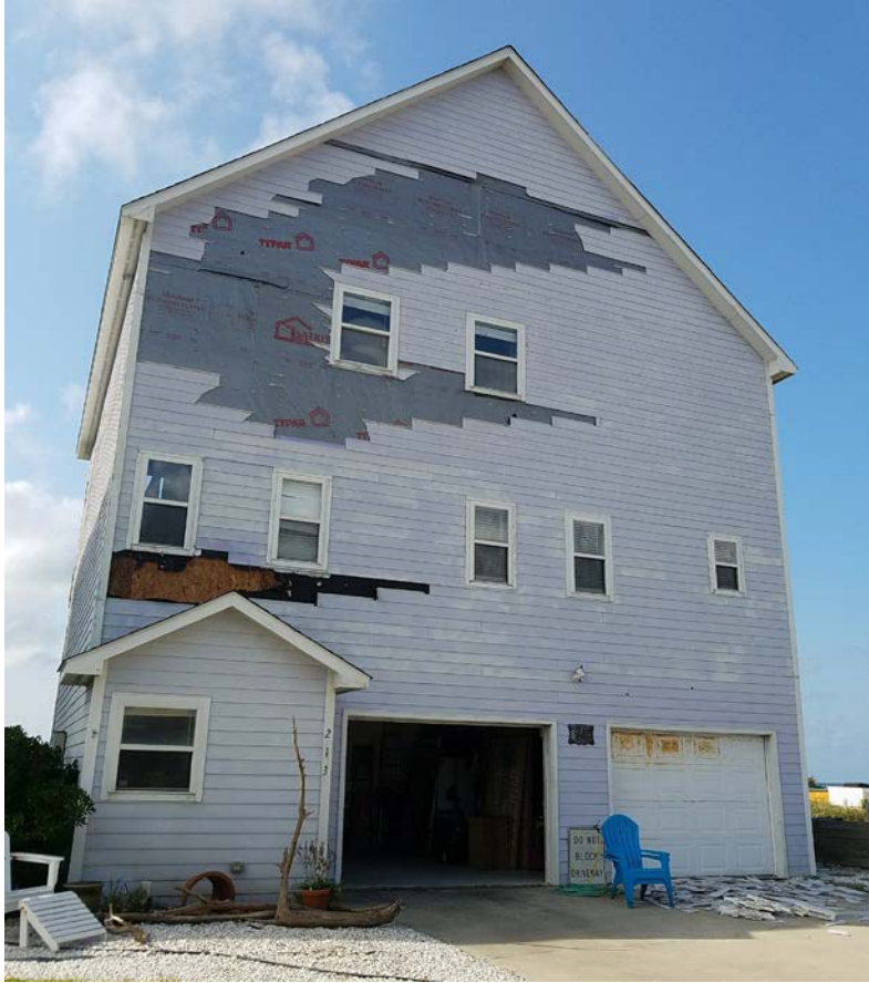
Figure 8: Loss of wall cover at residence in Atlantic Beach
