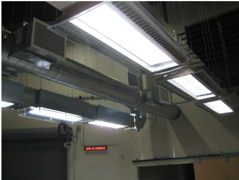
Reflective duct (the two ducts on the outside) in an open ceiling alongside a traditional HVAC duct.
