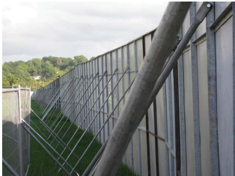
Fig. 10-4 - Solid temporary fence panels showing diagonal bracing. This is a pedestrian barrier used to channel queue lanes – perfect when no sideways pressure is anticipated. Photo courtesy of The Event Safety Shop, LTD.
