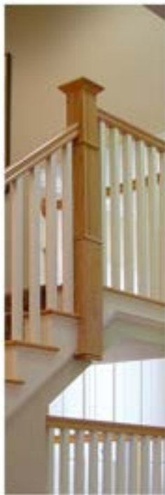
Handrail to Post as permitted by code
