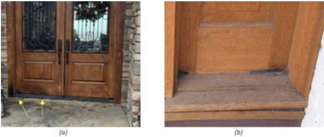
Figure 1. Ignition from accumulation of embers and debris at the base of the door.
