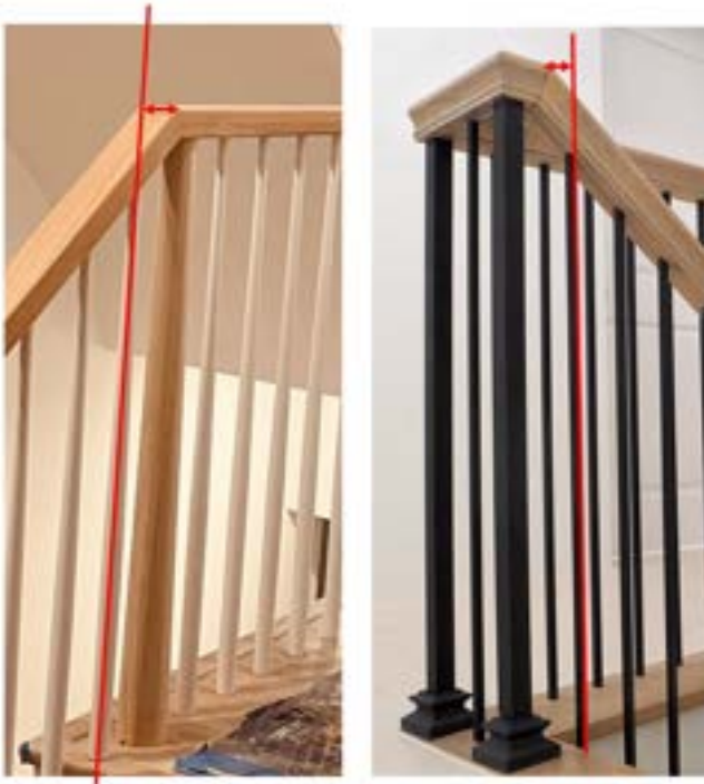
Simple Bisect of Handrail and Guard at Exactly Same Height The arrow indicates area addressed by new exception
