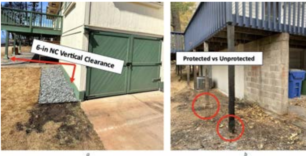
Figure 2. 6-in Noncombustible vertical clearance at the base of exterior walls and underfloor area columns: a. Lahaina Fire 2023 (Photo curtesy Milad Shobanian, IBHS), b. Glass Fire 2020 (Photo curtesy Steve Hawks, IBHS).
