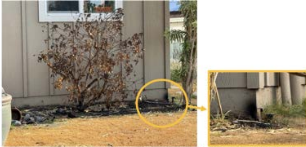
Figure 1. 6-in noncombustible vertical clearance worked as fuel break at the base of exterior walls in Lahaina wildfire. Photo credit: Steve Hawks, IBHS.
