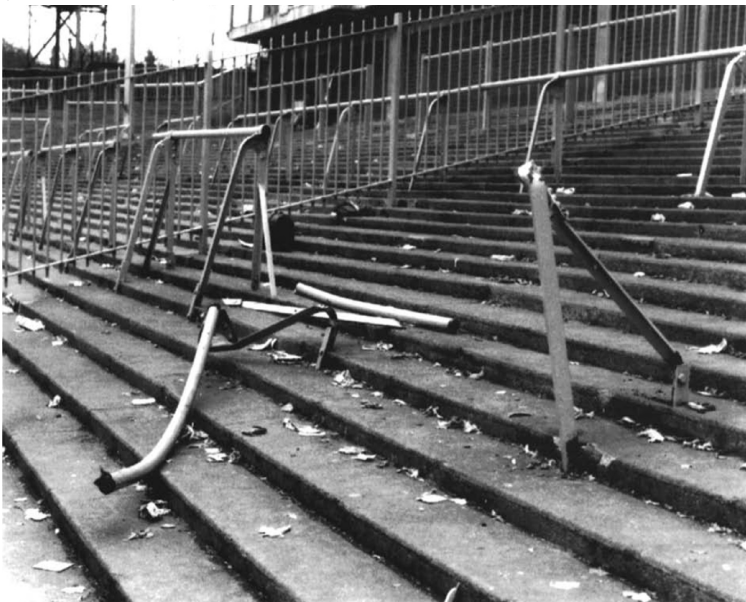
Figure 8: Hillsborough Braced railing collapse (Smith Report 1994)
