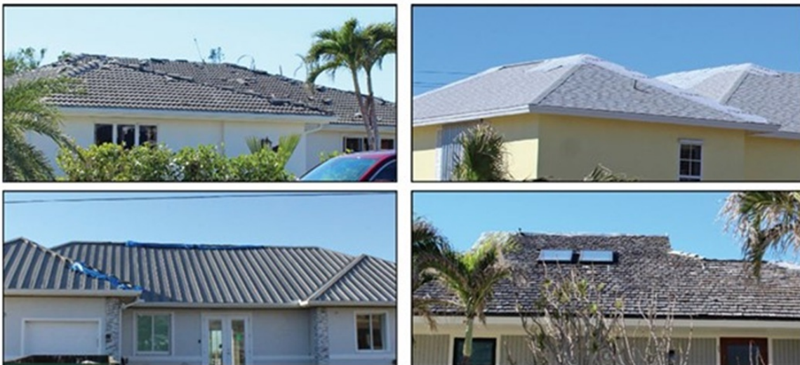
Figure 4-11: Hip and ridge damage on four residences with different roof types: a tile roof (top left), asphalt shingle roof (top right), metal panel roof (bottom left), and cedar shake roof (bottom right)
