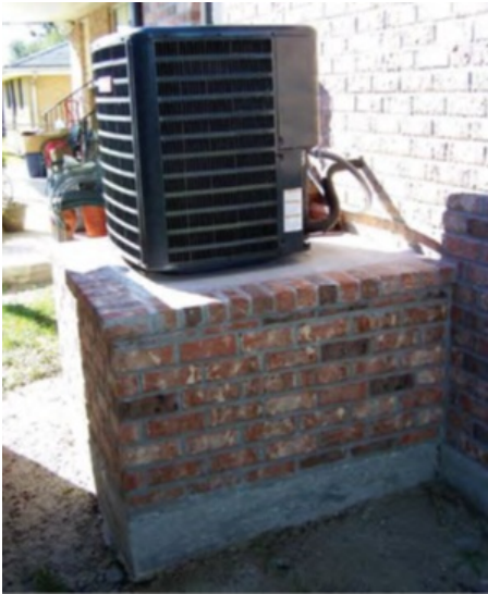
Equipment on platform
