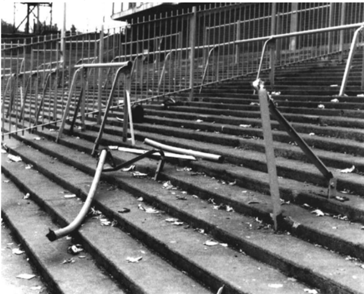
Figure 8: Hillsborough Braced railing collapse (Smith Report 1994)
