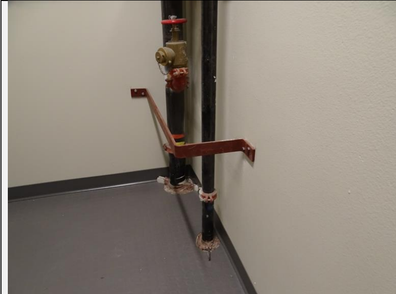
Example of a low bar. Detectable, but possibly an obstruction for general egress on the landing or could tangle with the hose. People with long canes are not typically using them in a stairway situation, so how much is this actually helping?
