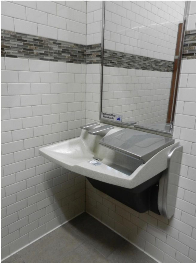
Hand dryer in the lavatory.
