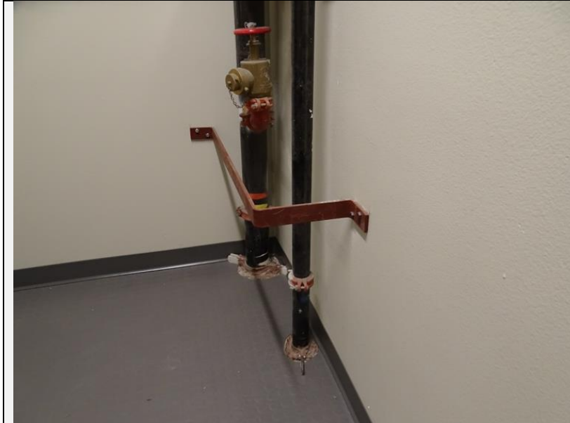
Example of a low bar. Detectable, but possibly an obstruction for general egress on the landing or could tangle with the hose. People with long canes are not typically using them in a stairway situation, so how much is this actually helping?
