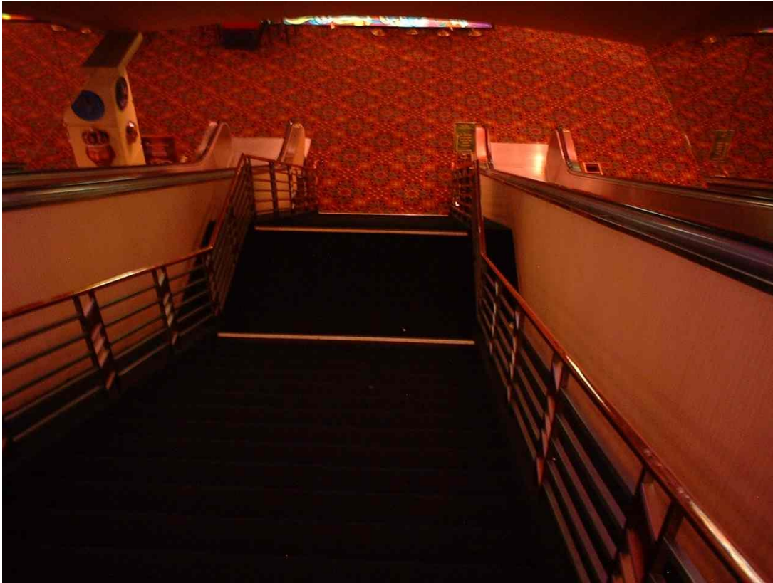
Examples of stairway markings in new exception.
