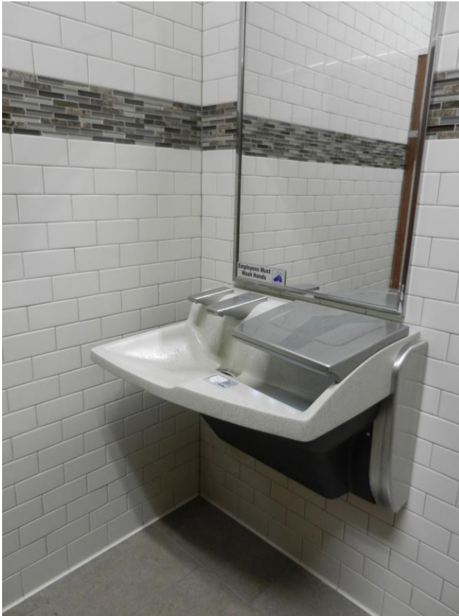
Hand dryer in the lavatory.
