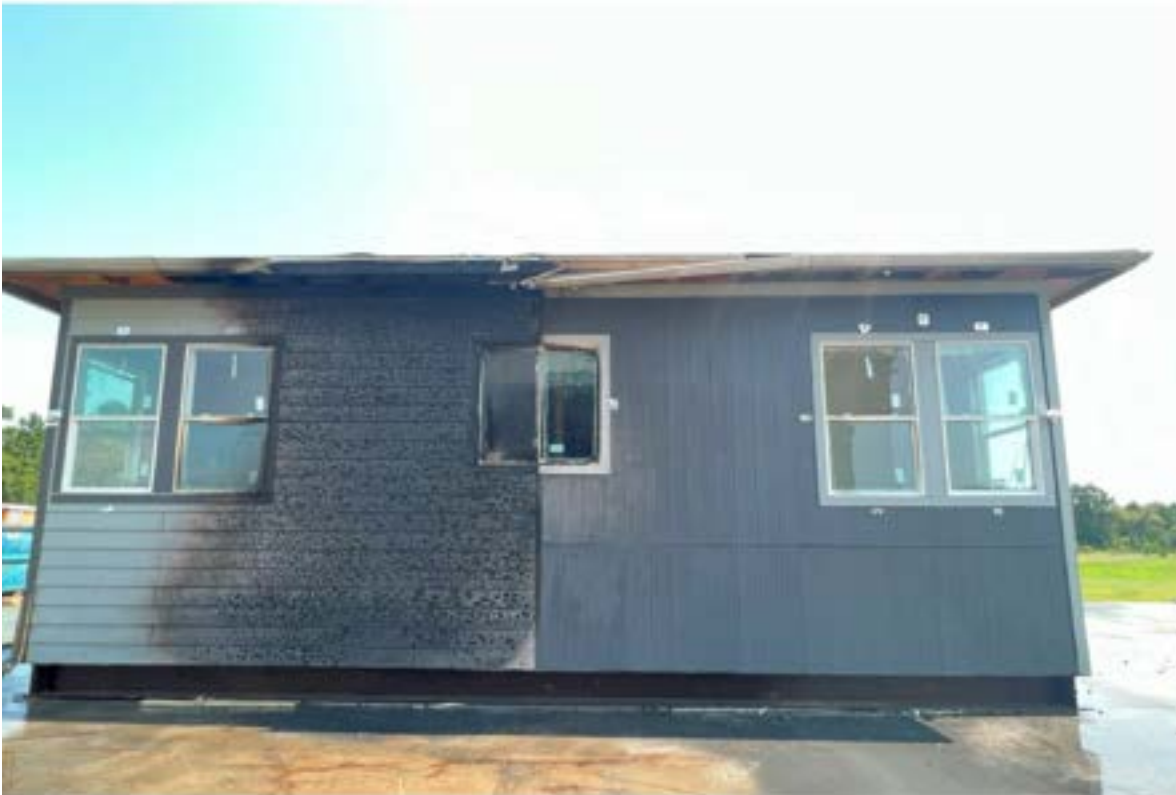
Figure 1. d. after suppression; severe damage can be seen on all components on the left-side.
