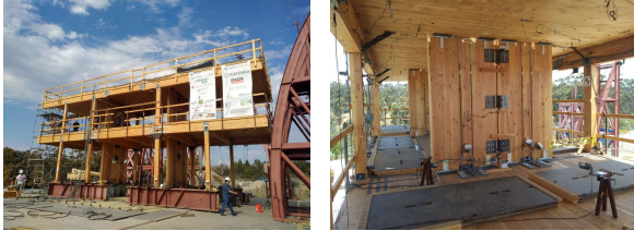
Photos Courtesy of NHERI Tall Wood Project, Photo by Dr. Shiling Pei at Colorado School of Mines
