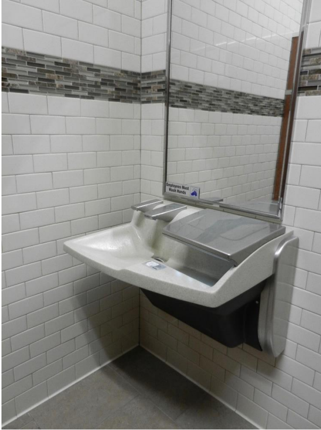
Hand dryer in the lavatory.
