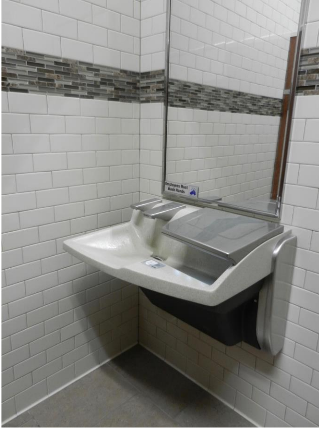
Hand dryer in the lavatory.
