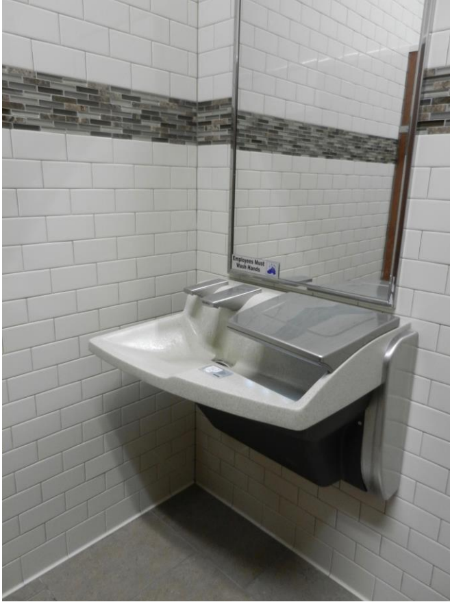
Hand dryer in the lavatory.
