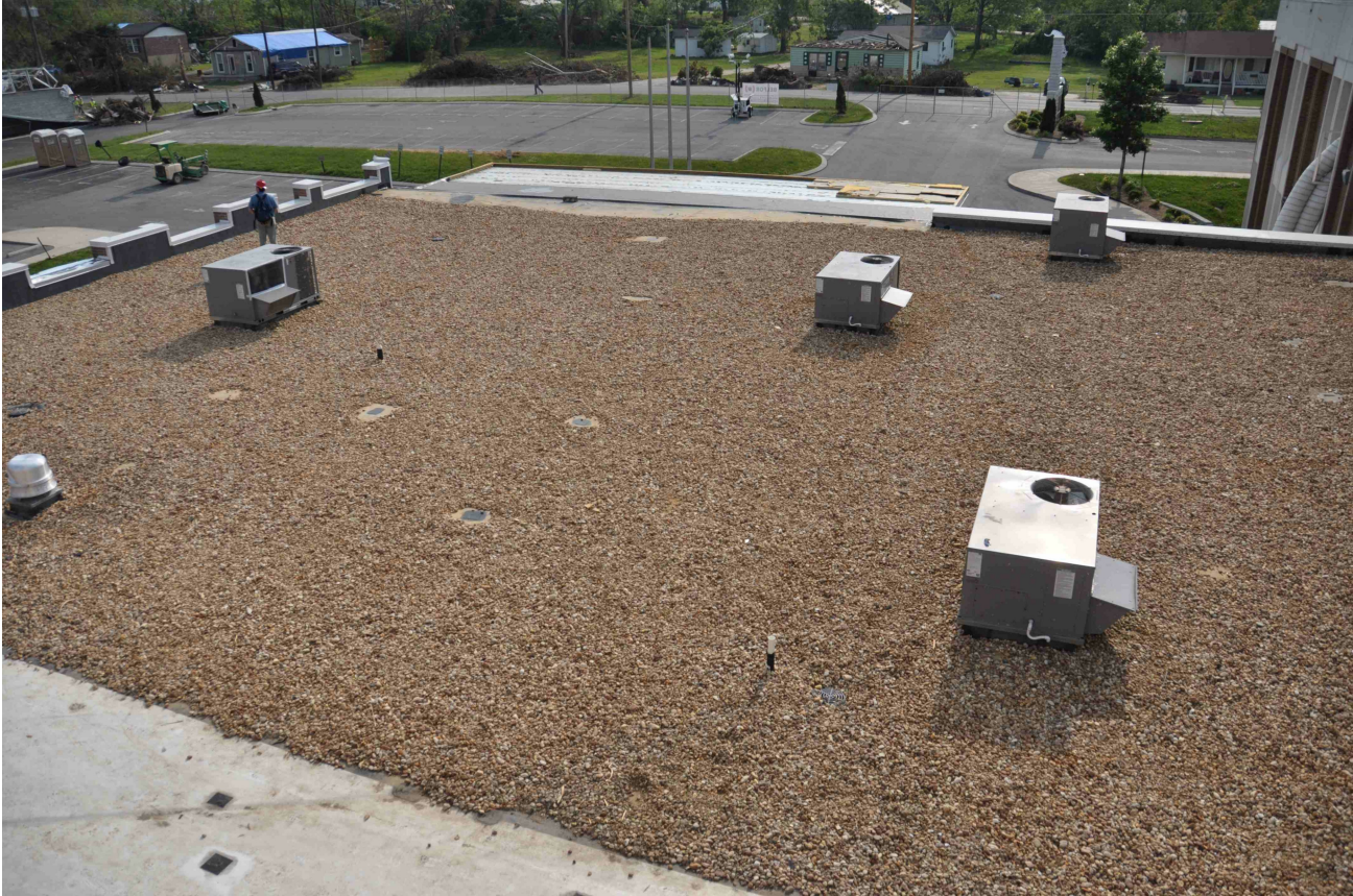
Figure 2a - Aggregate scoured from the roof of the first story section of this high school building in Georgia during a tornado (above) likely broke the windows on the adjacent taller section of the same building (below).
