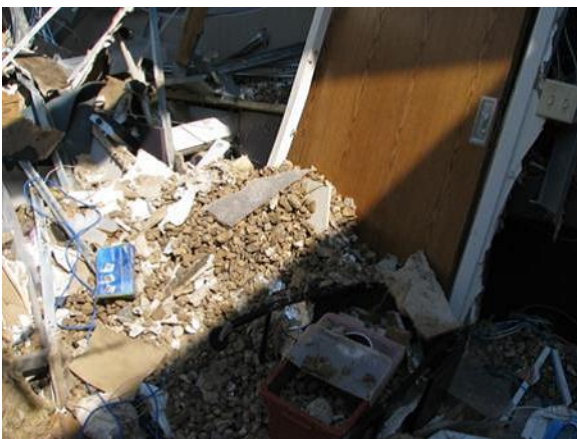
Figure 1b - Glazing failures in hospital tower at SJRMC following the Joplin tornado; interior damage at SJRMC. Note the extensive amount of roof aggregate inside the building.
