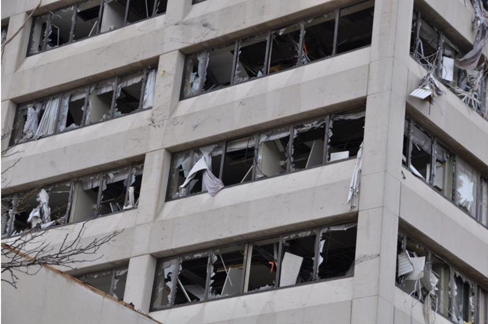
Figure 1a - Glazing failures in hospital tower at SJRMC following the Joplin tornado (above); interior damage at SJRMC. Note the extensive amount of roof aggregate inside the building (below).
