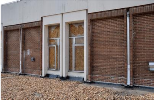
Figure 2b - Aggregate scoured from the roof of the first story section of this high school building in Georgia during a tornado likely broke the windows on the adjacent taller section of the same building.
