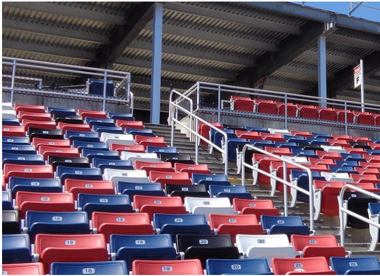
Figure 8 NASCAR Grandstand with mid-aisle handrail transitioning to handrails on each side where there are seats on neither side.
