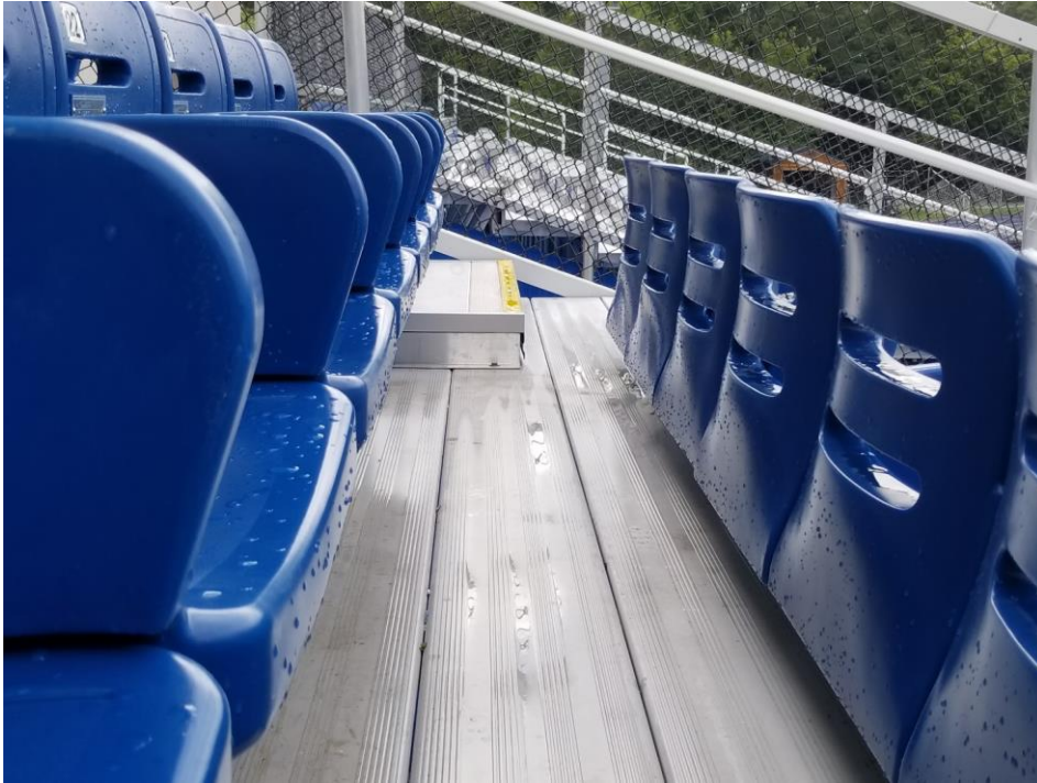
Possible tripping hazard at end of aisle accessway
