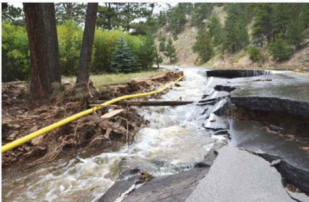
Damage in Coal Creek Canyon from the 2013 floods
